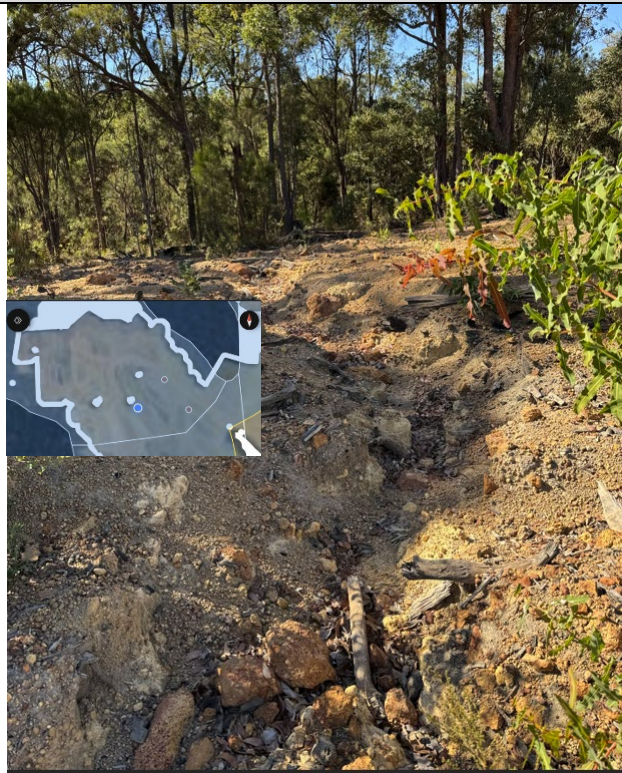
Erosion from the rehabilitate areas of Downes 10. Coordinates: (423,582E: 6,406,210N)
