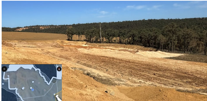
Drainage Control at Stone 13 drainage risk southern parts of the pit. Photo location (blue dot) is shown in the inset.
