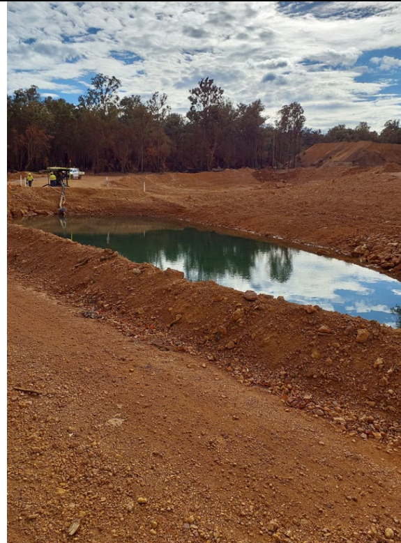
Sump at Macquarrie 1
