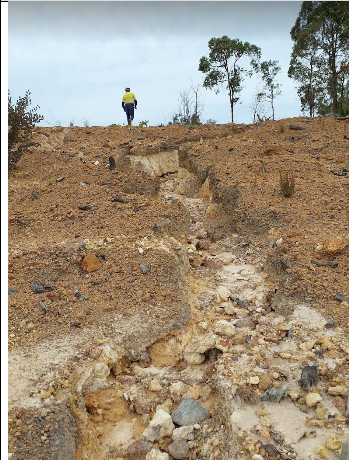
Erosion observed at Dellamaddalena 5 – photo from bottom of contour bowl looking up
