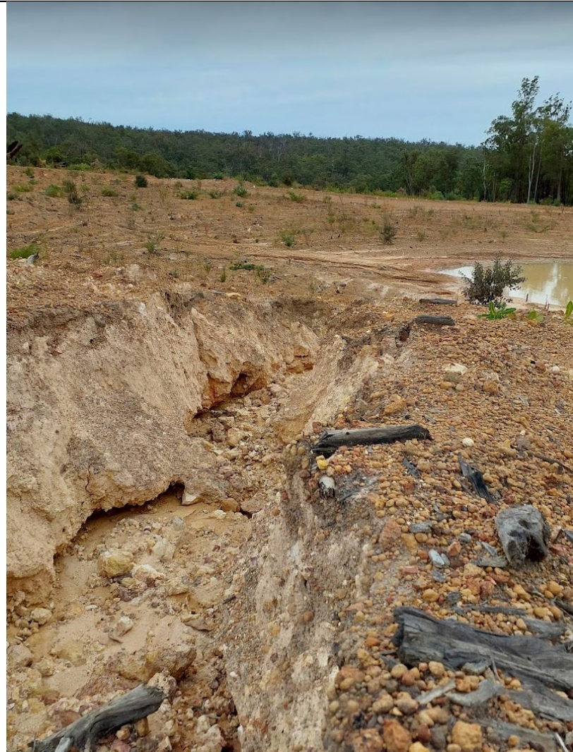
Erosion at Dellamaddalena 5 – looking down to pond in contour bowl. At this point the erosion was ~1m deep.
