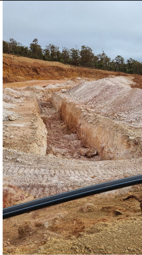
Mabbot 1 drain and pipeline installed for groundwater to be pumped up hill if necessary into upgradient drains.
