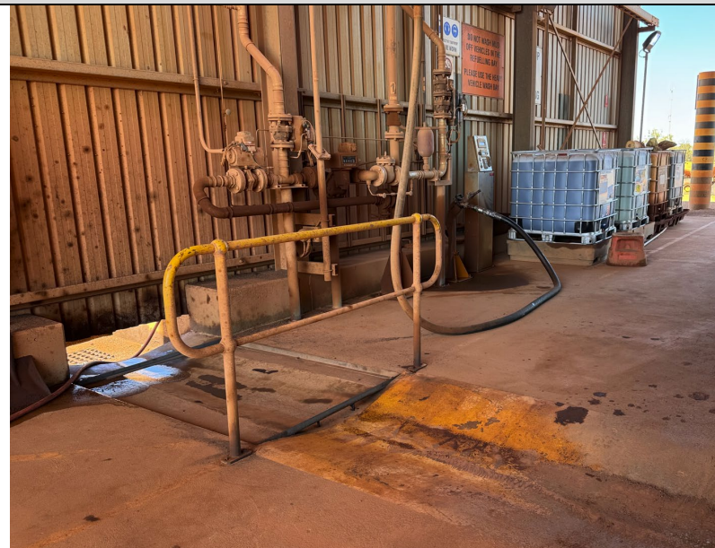
Heavy vehicle fuel farm drainage channels for fuel spill
