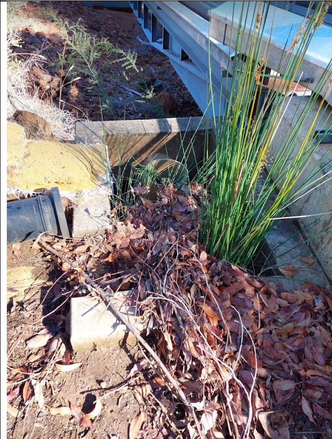
AOI - Samson Dam crossing area stormwater capture point filled with leaves
