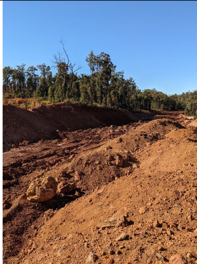
Gibber 10 - ripping through road leading to forested area to prevent water entering rehabbed areas.
