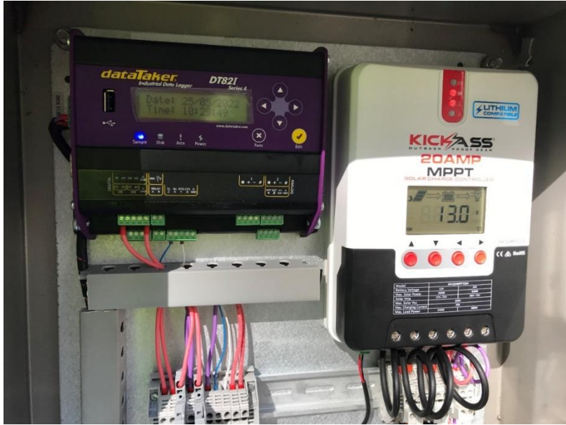
Figure 2. Turbidity data logger interfaced with stream channel monitor.
